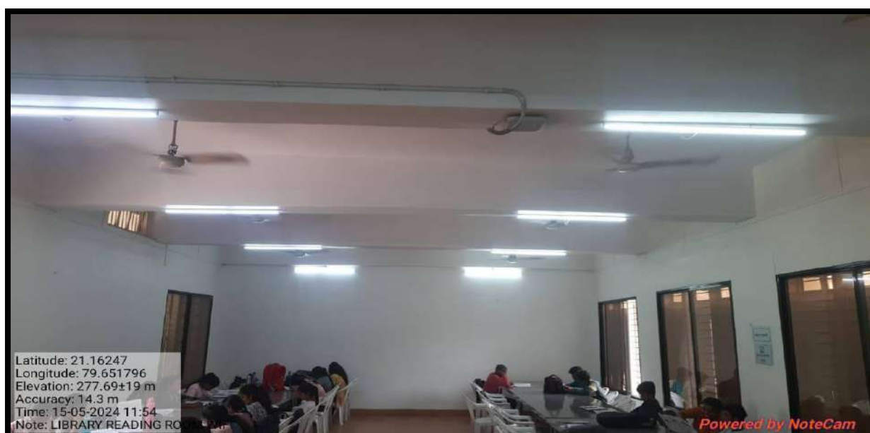
LIBRARY READING ROOM WIFI ROUTER - 5
