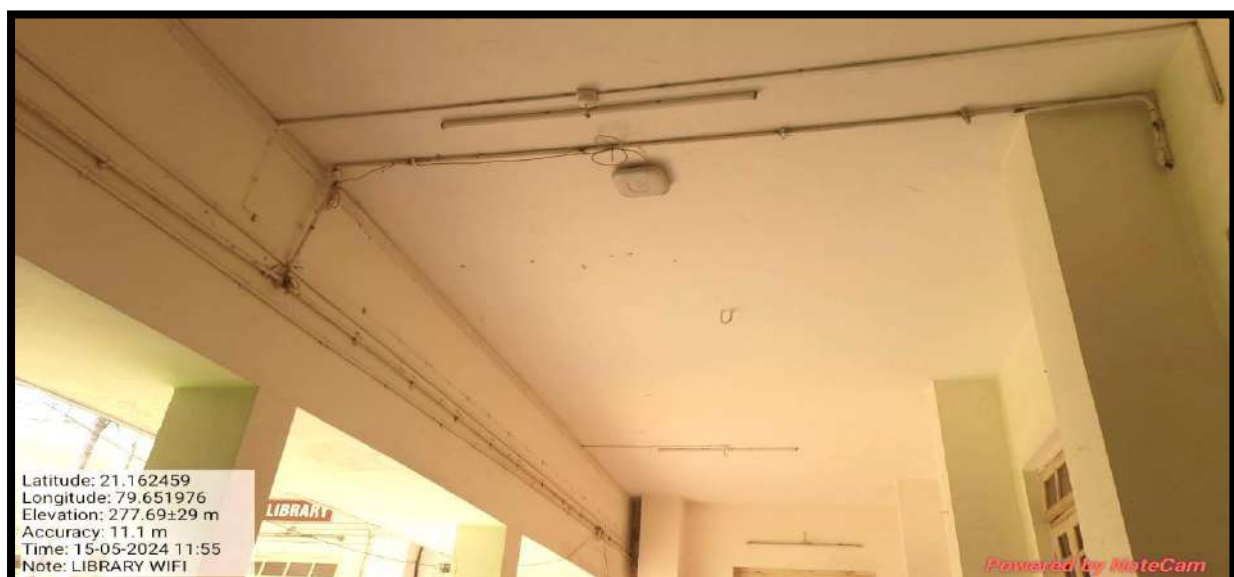
LIBRARY WIFI ROUTER - 3
