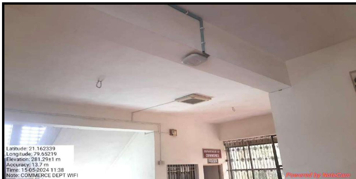
COMMERCE DEPARTMENT WIFI ROUTER - 7
