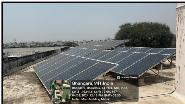
Rooftop Solar Power plant - Main Building
