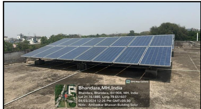
Rooftop Solar Power plant – Ambedkar Bhawan
