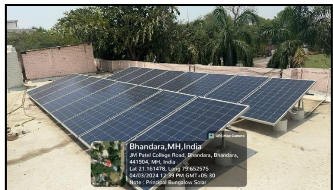
Rooftop Solar Power plant–Principal Bungalow
