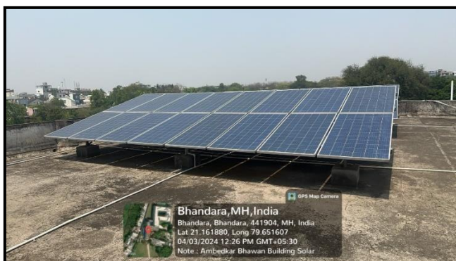
Rooftop Solar Power plant - Science Building
