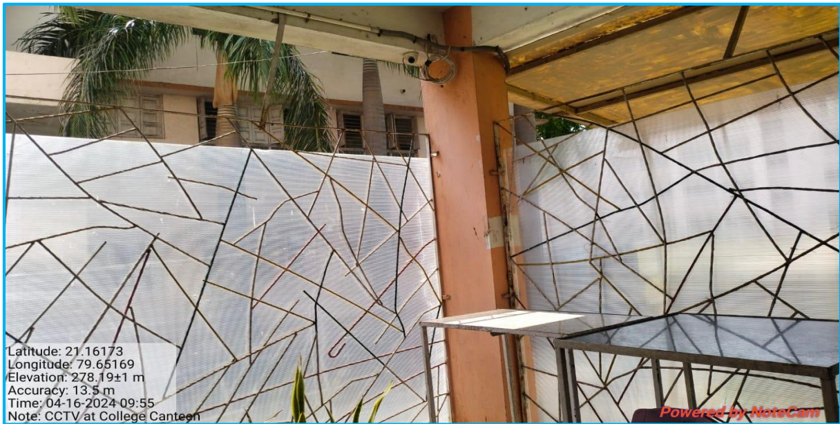
Camera installed at the Canteen for safety of girls
